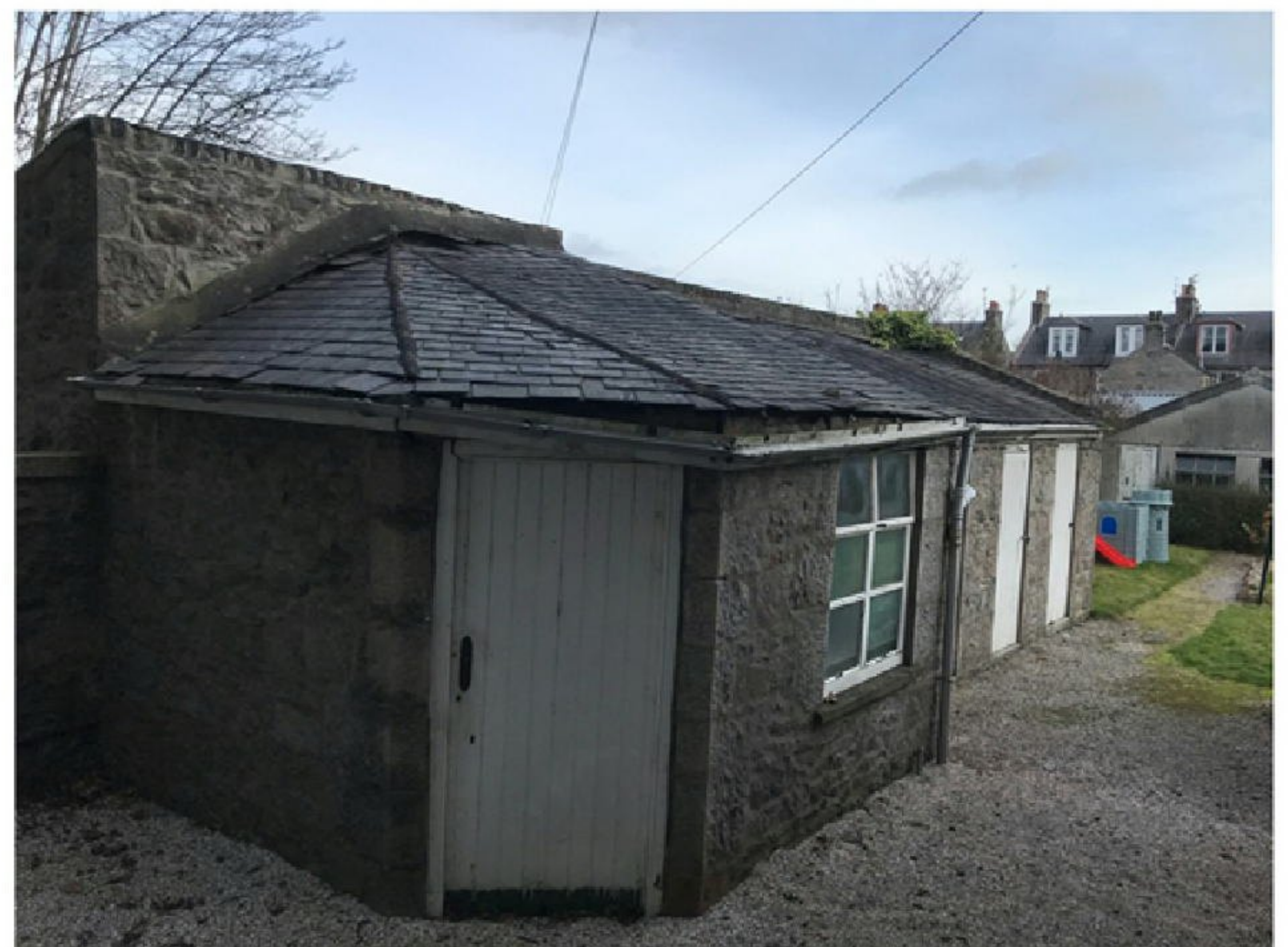
Photo 06. The existing washhouse taken from the back door of 18 Fountainhall Rd. The building is derelict and redundant and has been unused for in excess of 20 years.
